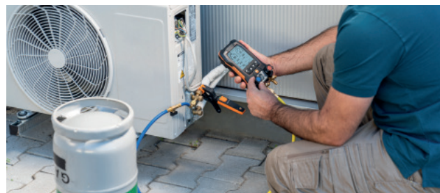
testo 550s digital manifold and testo 115i smart probe being used to service an air conditioning unit.
